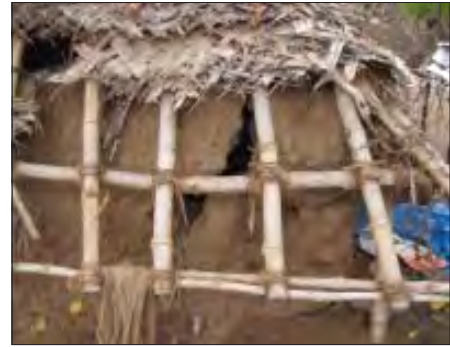
Damaged Wall and Roof
