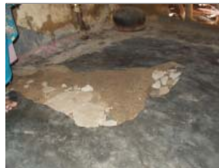
Damaged Flooring Material
