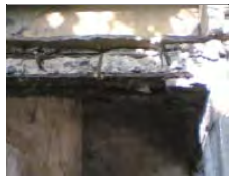
Damaged Roof Beam
